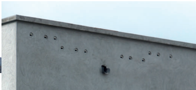
Built-in Schwegler 17a nest boxes at Westport Town Hall, Co. Mayo
